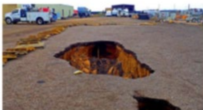
The reactivated fissure immediately north of W. Houston Rd. in July 2017, was approximately 0.75 miles in length AZG Library
